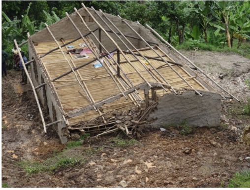
Family house that collapsed
