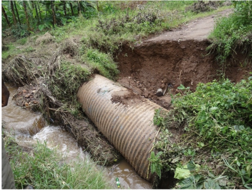
Community road and bridge destroyed
